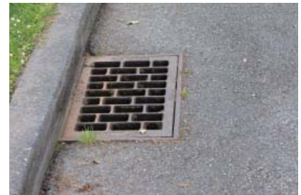
Catch basins for current storm water system.
