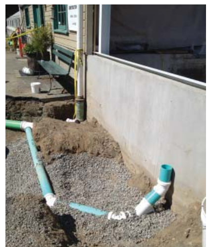
Storm water sewer system.
